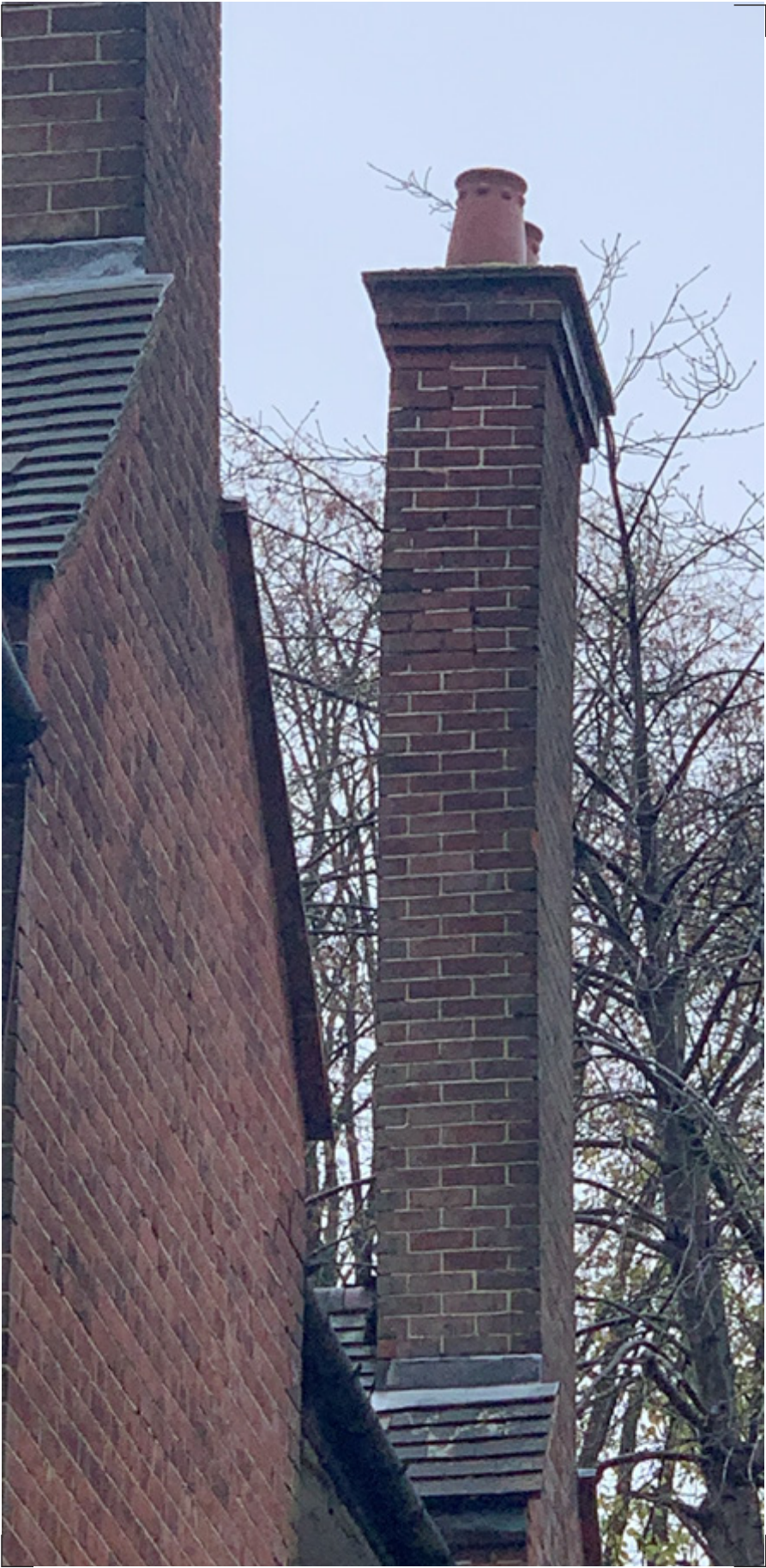
EXISTING CHIMNEY POST STORM.
