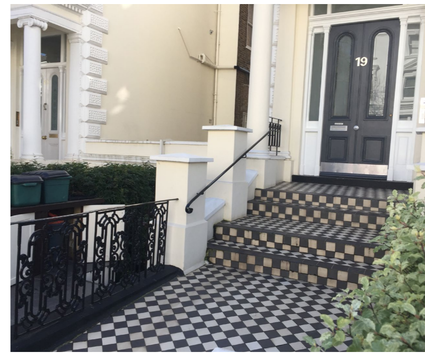
No. 19 Belsize Park Gardens (simple railing only along the stairs, as proposed for No. 17)
