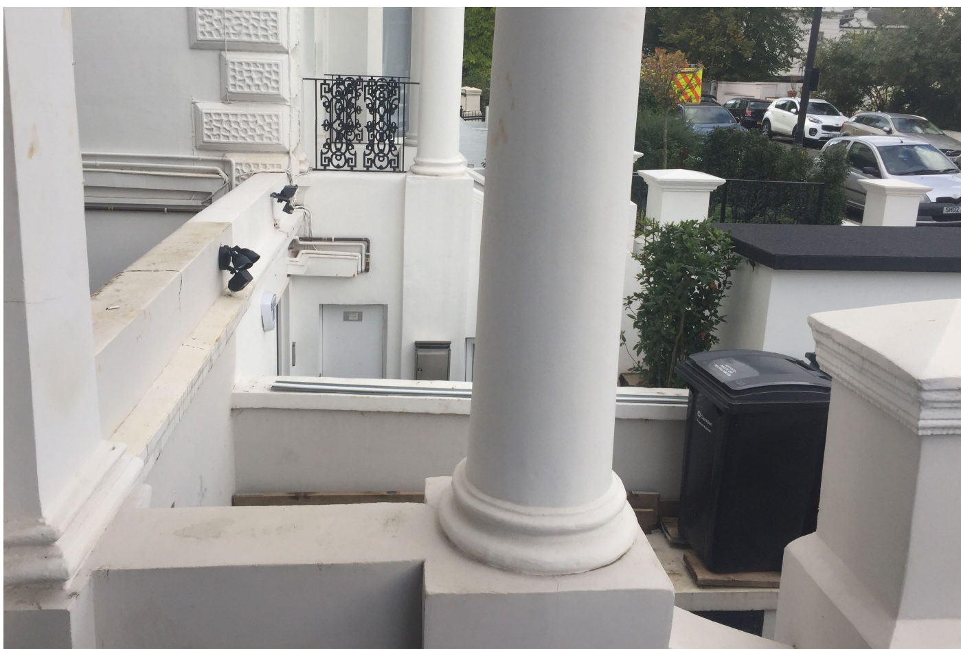
PHOTO 3 - No parapet or handrails between piers across the staircase
