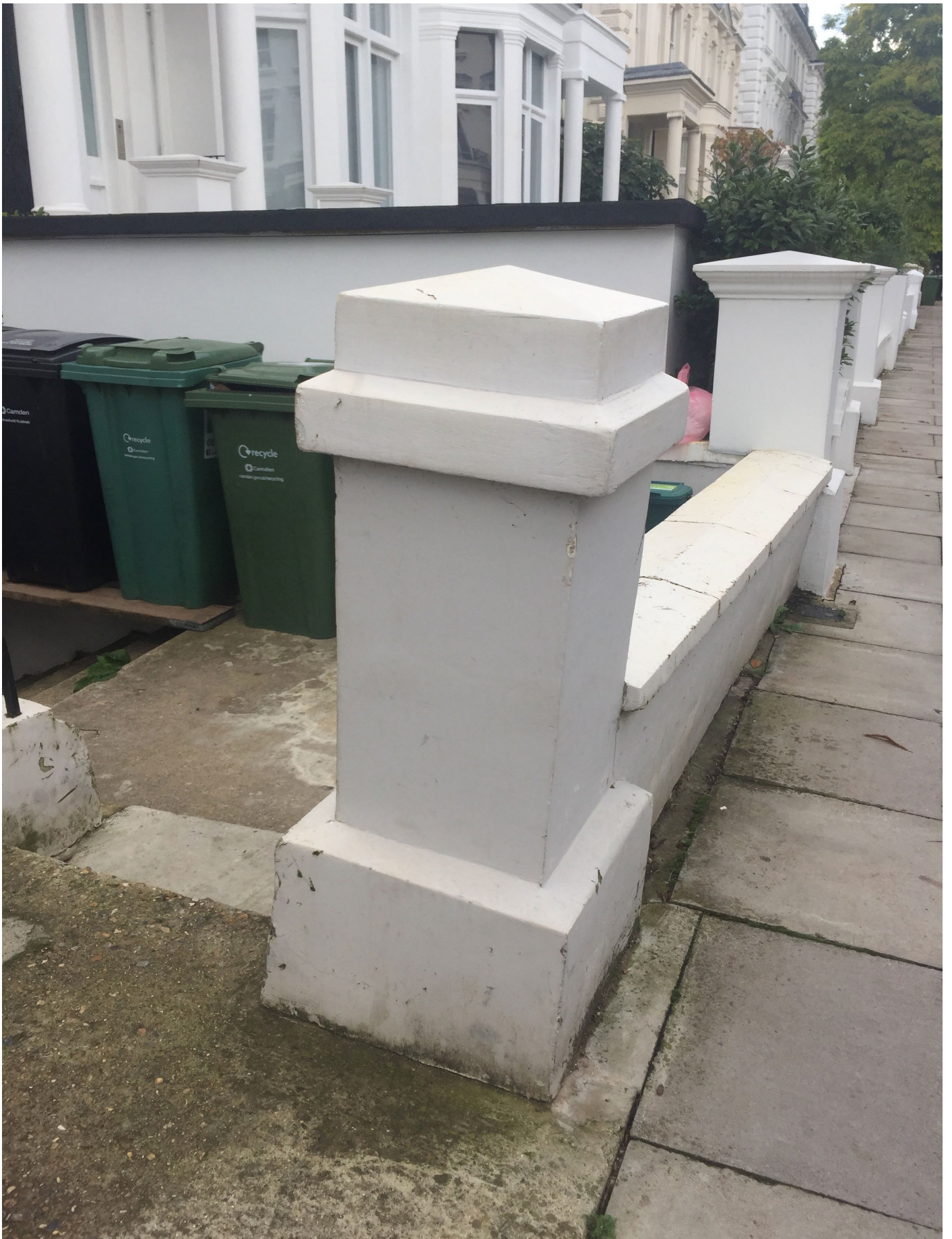
PHOTO 1 - Leaning pier and parapet wall
