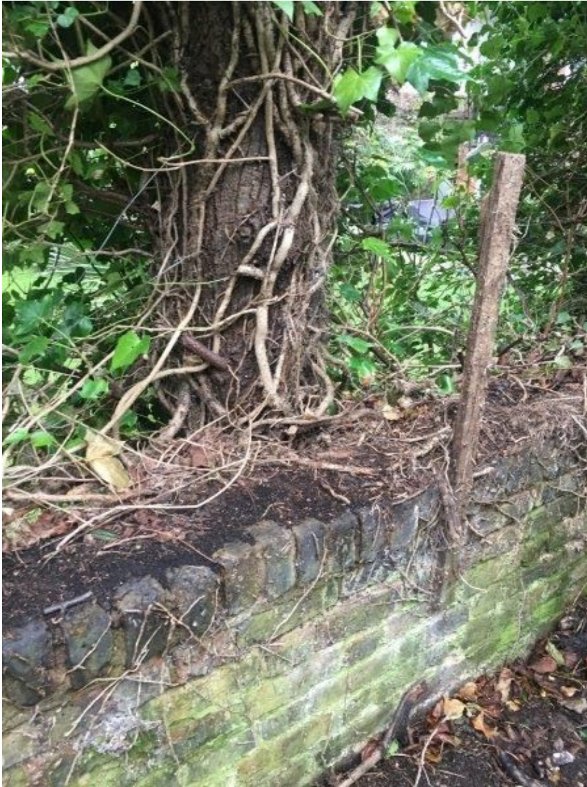
Photo 4: T2 trunk against boundary wall
