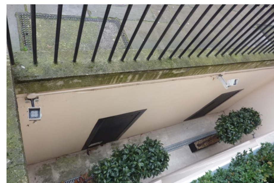
EXISTING PLANT LOUVRES IN NO. 37 CHESTER TERRACE FRONT LIGHT WELL TO BE ENLARGED
