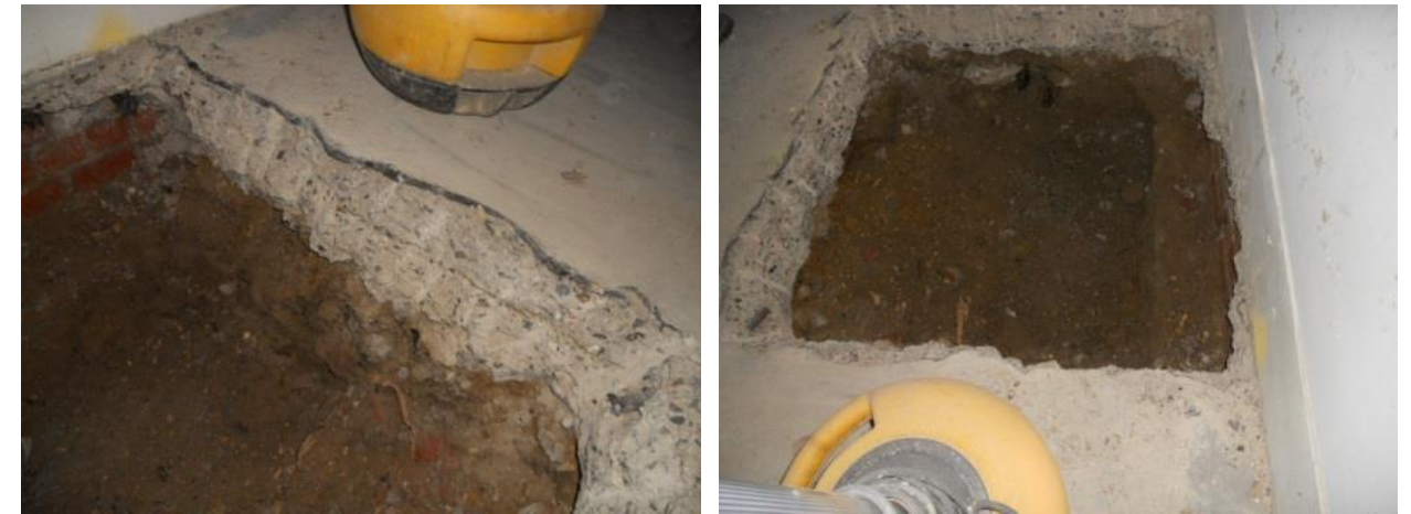
Figure 30: 2010 trial pit in Lower Ground Floor of No. 36 Chester Terrace shows non-original concrete slab and tanking.
