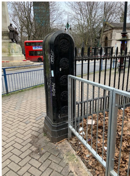
Original cast iron railings and pillar to be replicated. New metal utility railings abutting pillar
