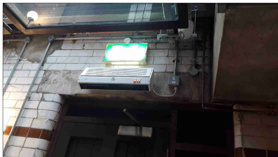
Typical emergency lighting
