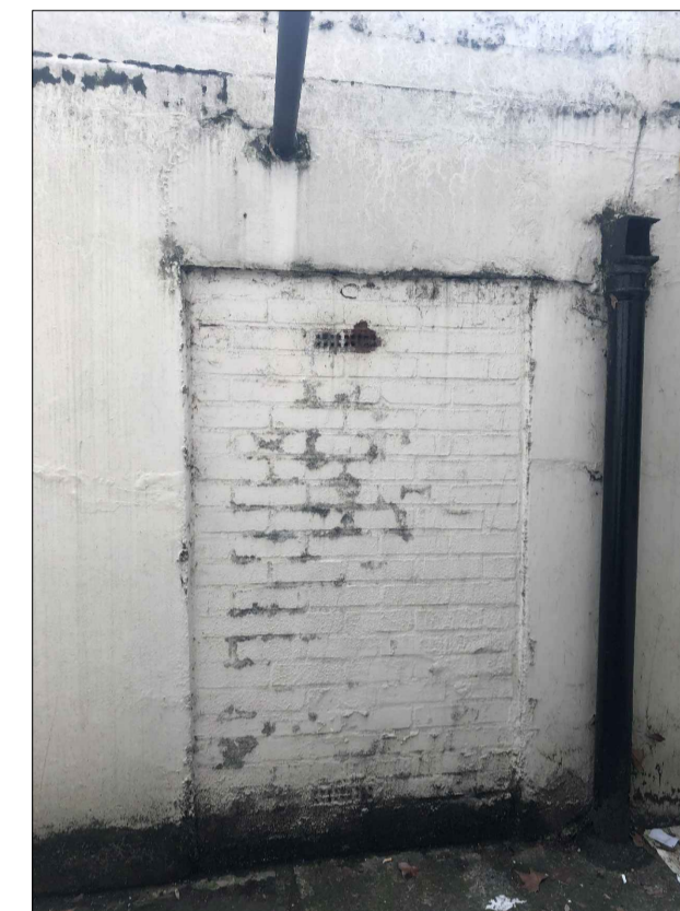
Typical blocked vault opening
