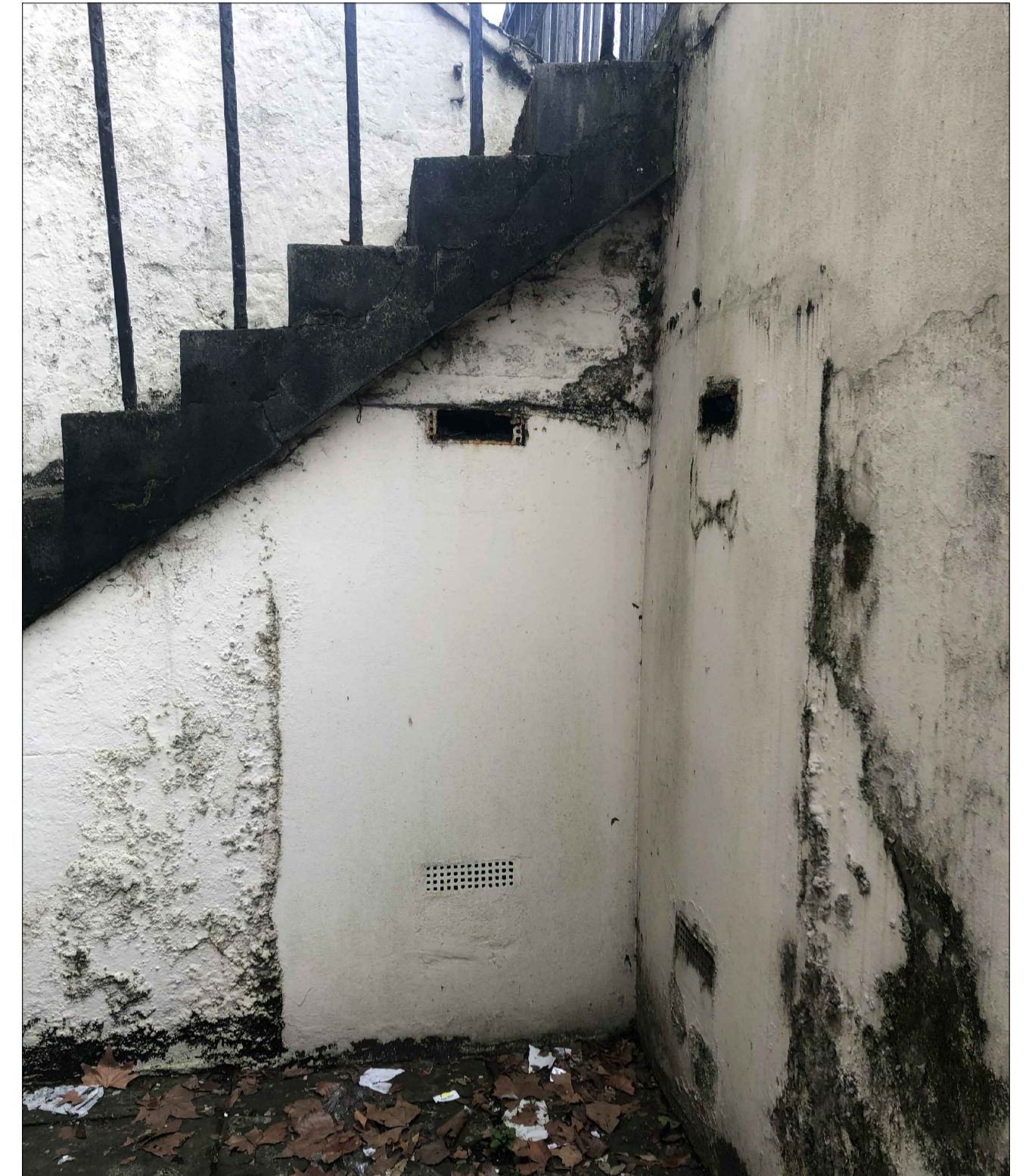
Photo showing typical condition of blocked opening
