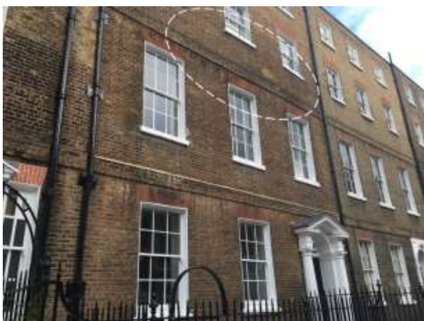
Fig.03 Detail indicating location of delamination
