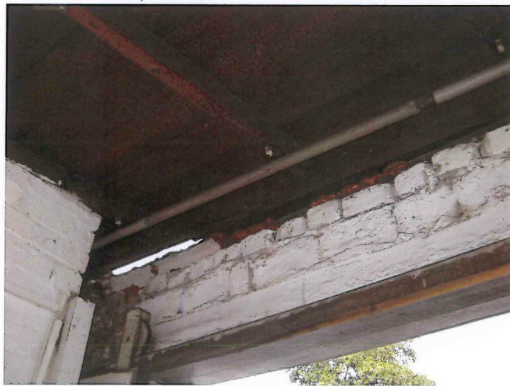
Plate 3: Brick above timber lintel to front not tied to timber roof
