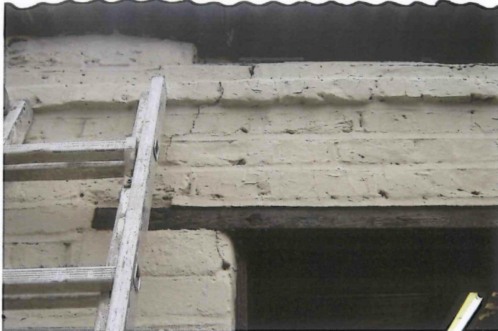
Plate 6: Crack to LHS above timber lintel bearing
