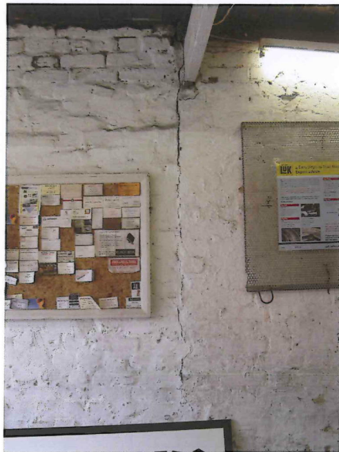
Plate 5: Vertical crack to left hand side flank wall
