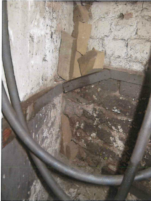
Plate 7: Vertical crack at junction of rear wall and return wall
