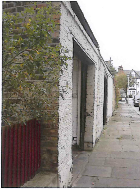
Plate 2: Central brick pier leaning outwards at top
