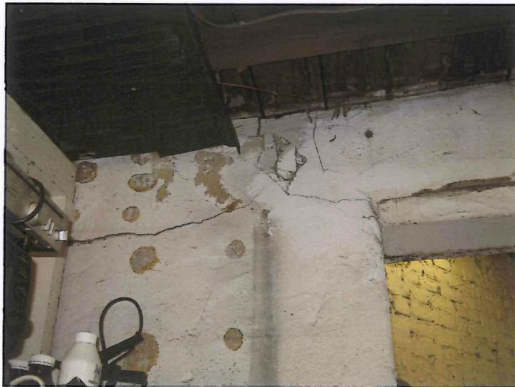
Plate 4: Crack to rear brick pier
