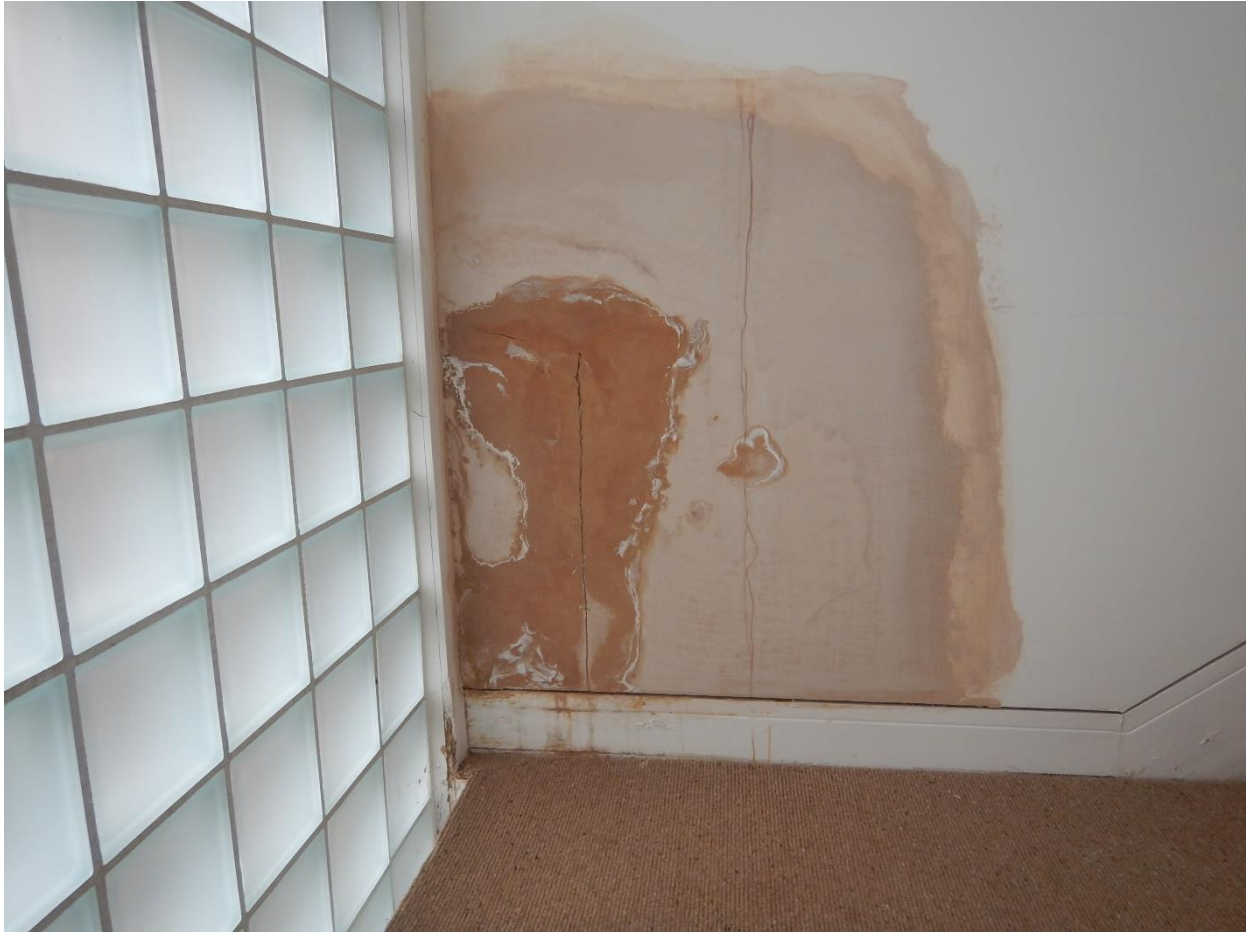
Figure 26. Damage from damp is visible within the interior spaces of the house.
