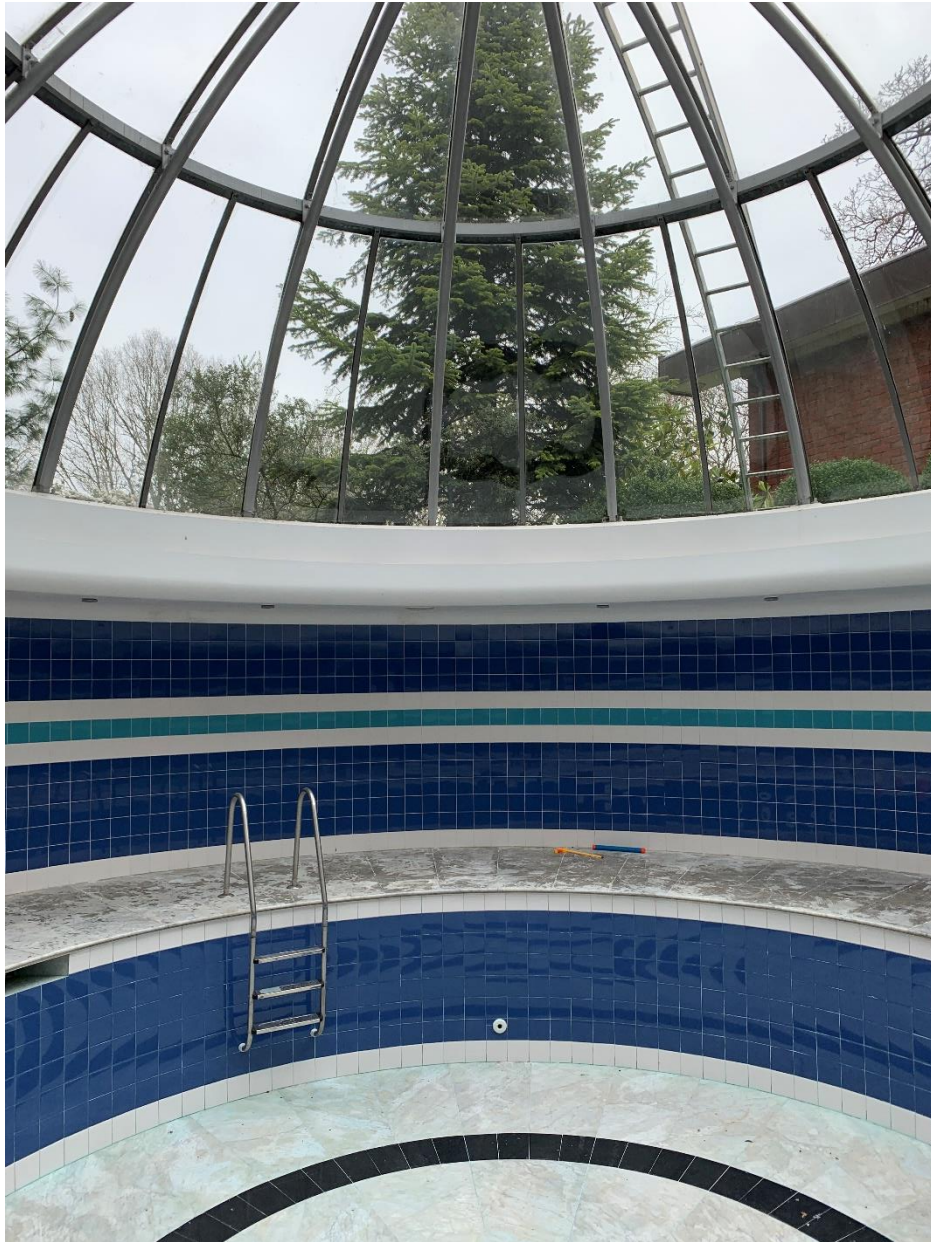
Figure 19. View of pool showing replacement tiles to the surrounding walls, and marble finish to pool floor.
