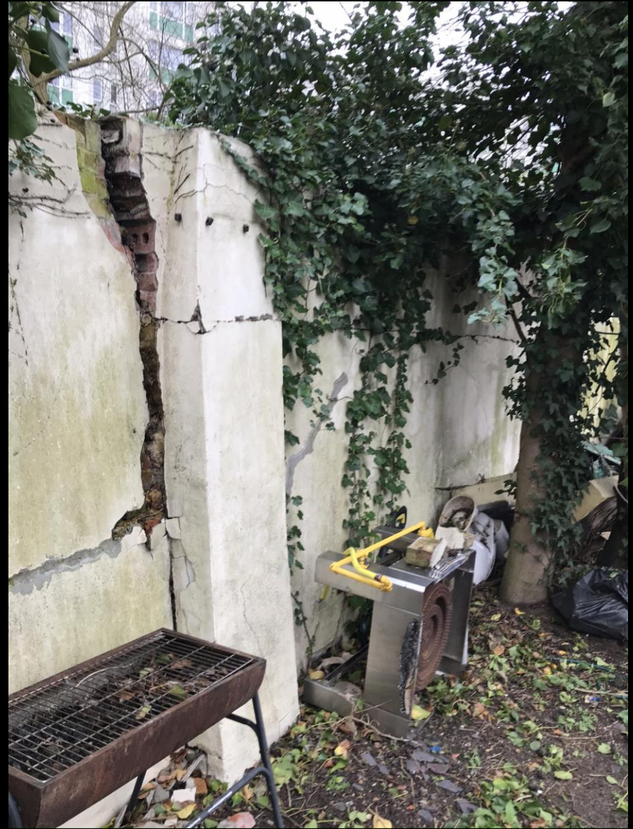
Poor condition of wall near trees T3 and T4.
