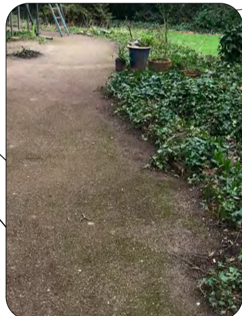
Existing red asphalt paths to be refinished with quarry tiles - see proposed plan drawing (PL)25.
