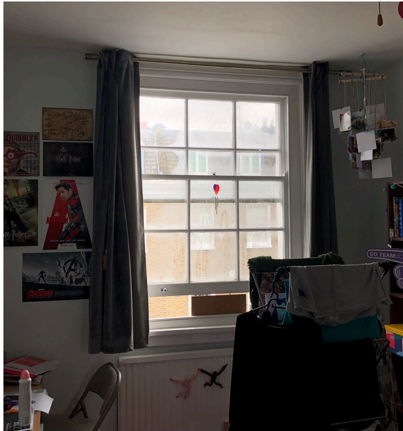
Figure 8: Internal view of window at second floor level – Bedroom C (Flat C)
