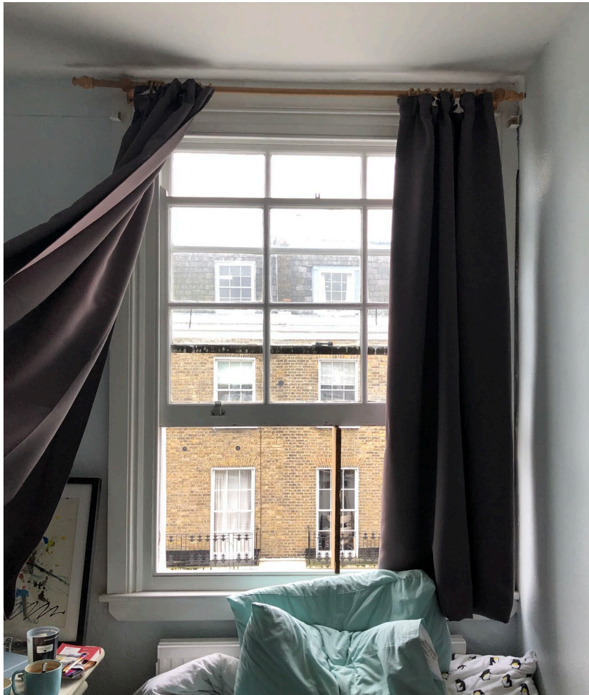
Figure 7: Internal view of window at second floor level – Bedroom B (Flat C)
