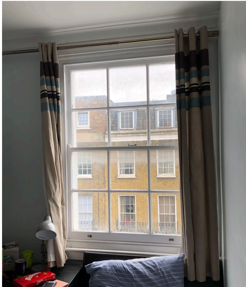
Figure 6: Internal view of window at second floor level – Bedroom A (Flat C)
