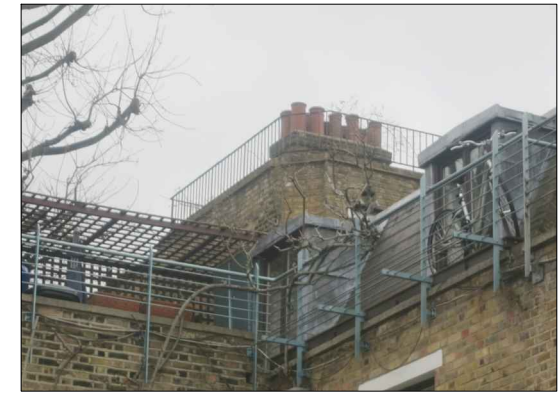
3. REAR ELEVATION OF ROOF EXTENSION INCORPORATING A ROOF TERRACE WITH PERIMETER RAILINGS - NEIGHBORING PROPERTY
