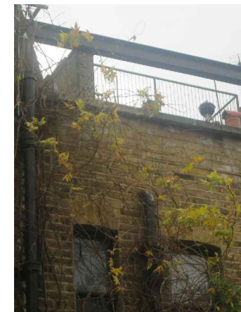
6. REAR ELEVATION OF ROOF EXTENSION INCORPORATING A ROOF TERRACE WITH PERIMETER RAILINGS - NEIGHBORING PROPERTY
