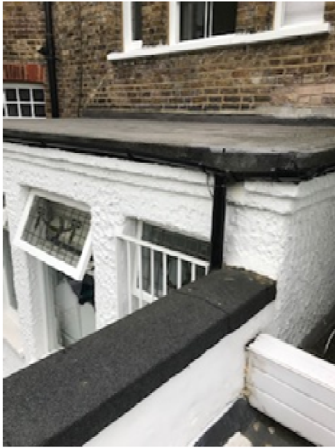
7. Views of the windows on the rear elevation of the ground floor flat from the existing conservatory
