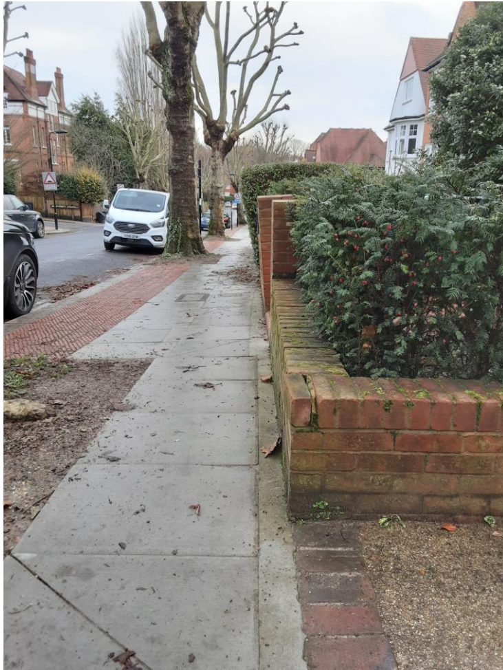
Photo 3: Brick pillar leaning towards pavement
