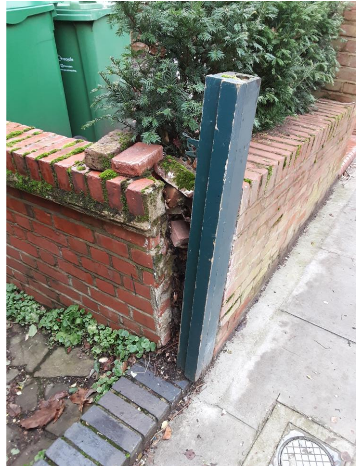
Photo 2: Damage to neighbours gate post and wall
