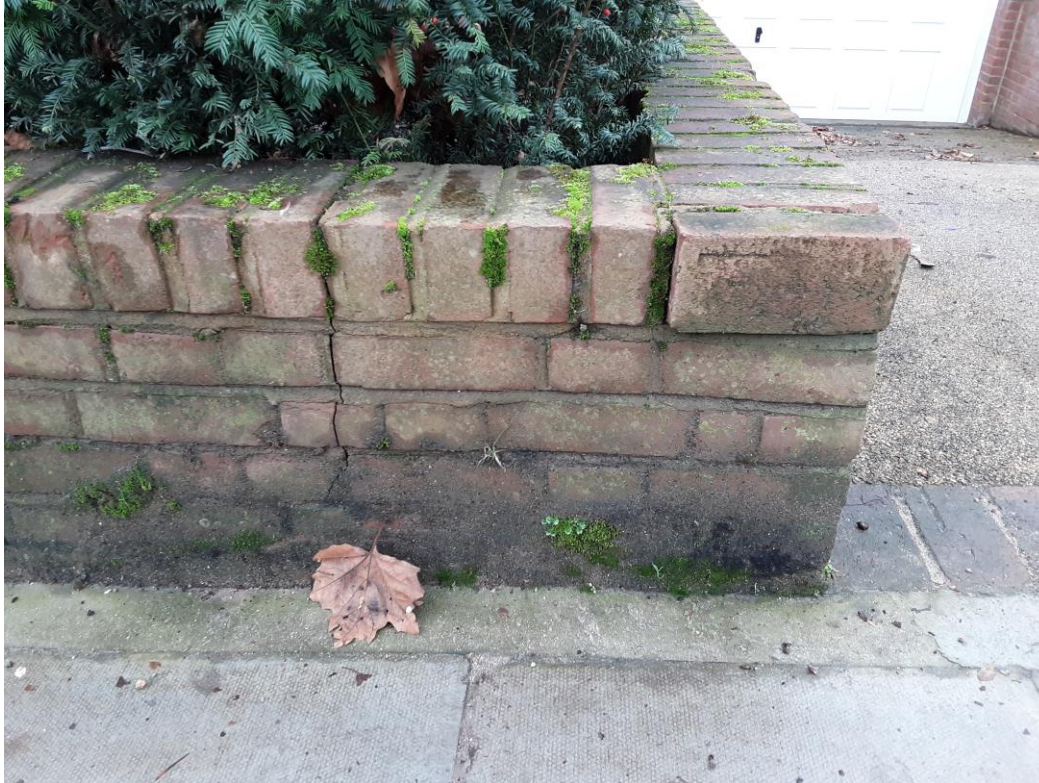
Photo 5: Cracking of wall corner
