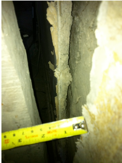
Photo No. 12 Movement of the internal face of the end gable wall and the final timber stun in the spine wall.
