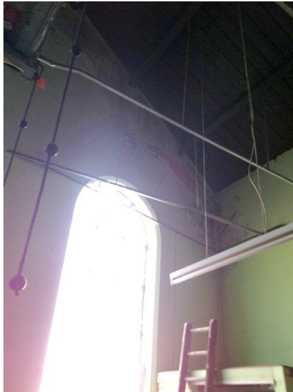
Photo No. 10 Cracking at front south wall junction.
