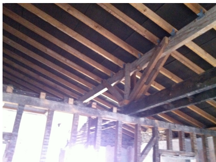
Photo No. 8 View of rear elevation showing distortion inwards above first floor level.
