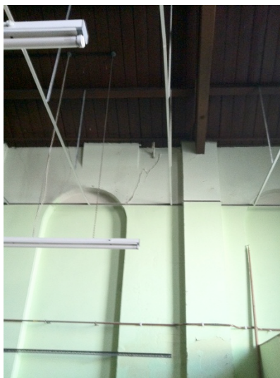
Photo No. 6 Internal detail of South facing flank wall, at junction with front wall. Note crack in flank.
