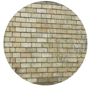
Brickwork to match
