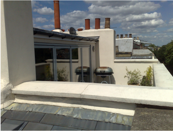
Existing view from the roof of No. 38 looking towards the recently completed roof extension at No. 36 England's Lane.
