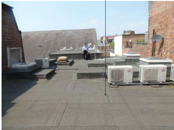
Right: Flat roof level view looking to the west side of the site (Grafton Yard)
