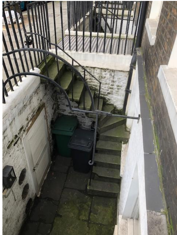
Photograph 4: Existing concrete staircase to the front elevation lightwell of 49 Doughty Street. It is proposed to replace this with a new cast iron and mild steel staircase.
