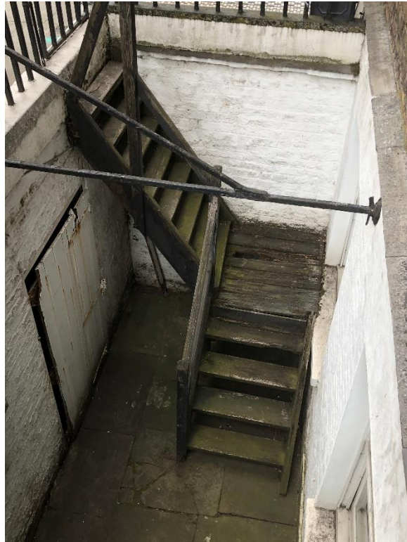
Photograph 3: Existing timber staircase to the front elevation lightwell of 48 Doughty Street. It is proposed to replace this with a new cast iron and mild steel staircase.
