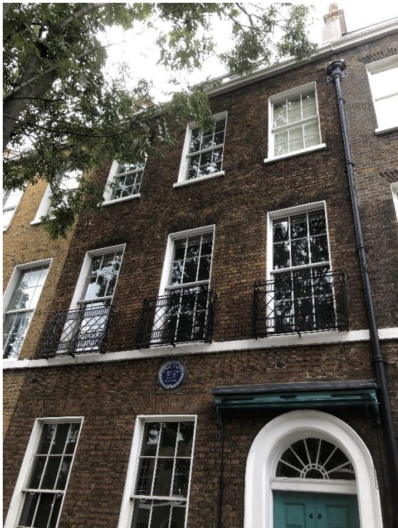
Photograph 2: Photograph showing the existing downpipe and hopper to the front elevations of 48 & 49 Doughty Street. The 2no. proposed overflow pipes will be installed above the cornice visible above the hopper.
