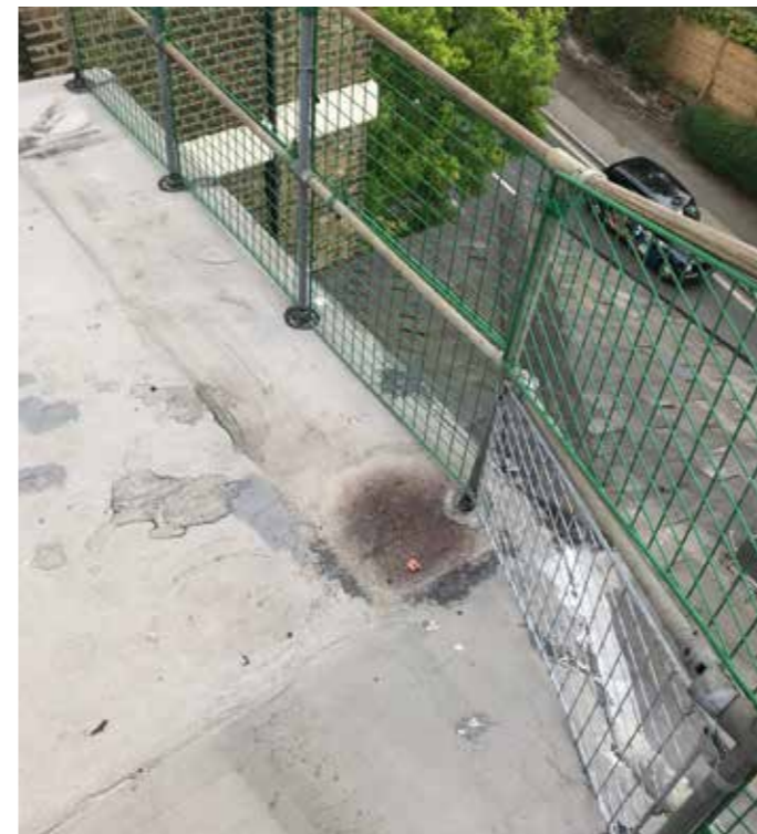
Industrial balustrade and fall protection. High water egress risk and damage to roof covering
