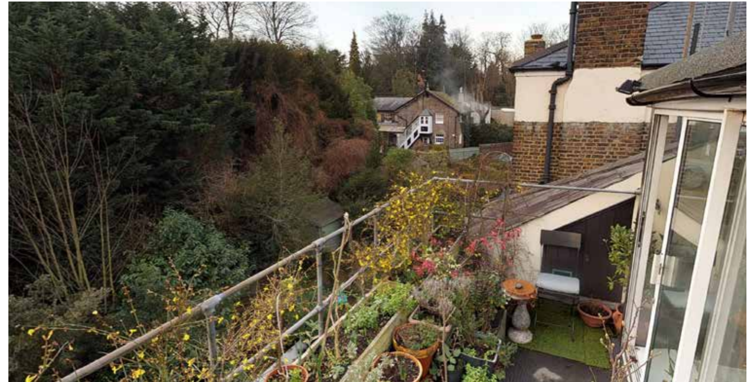
Rear Terrace and extension - Dilapidated and unsightly materials and execution
