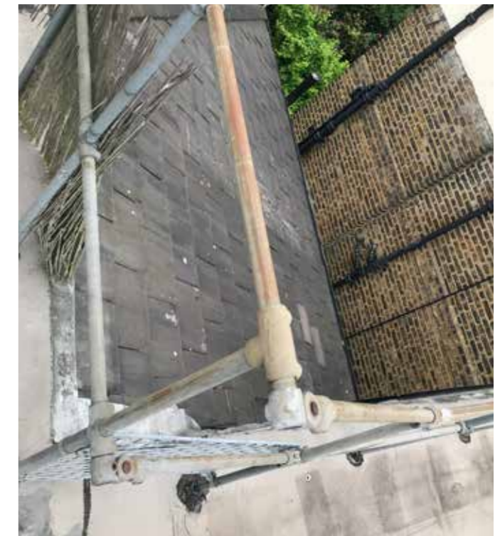
Industrial balustrade with no fall protection provided
