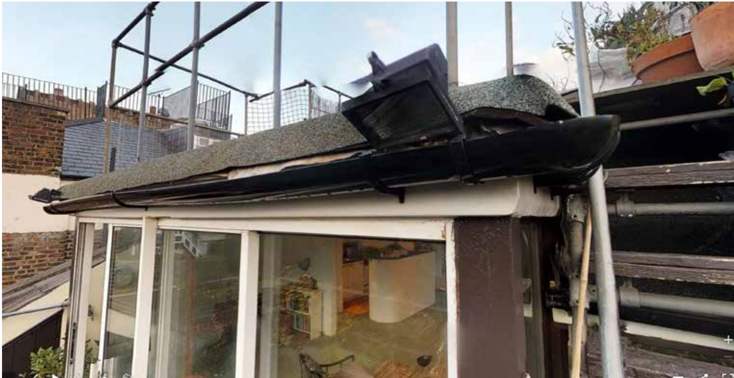
Rear Terrace and extension - Dilapidated and unsightly materials and execution
