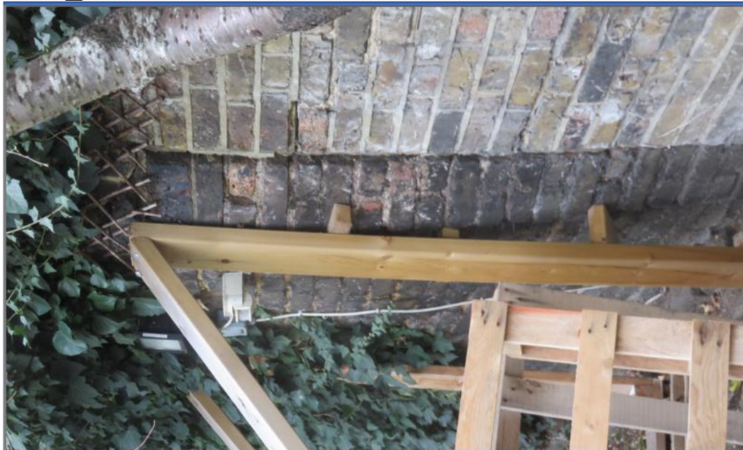
IMG_6128 Side shot of wall showing bulge
