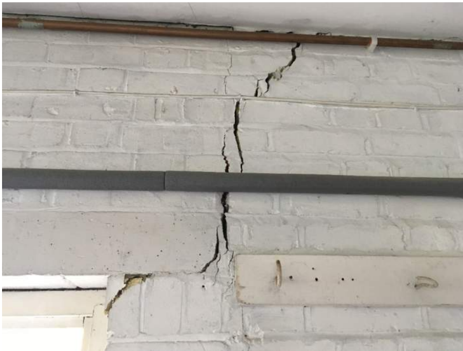
Damage in Garage
