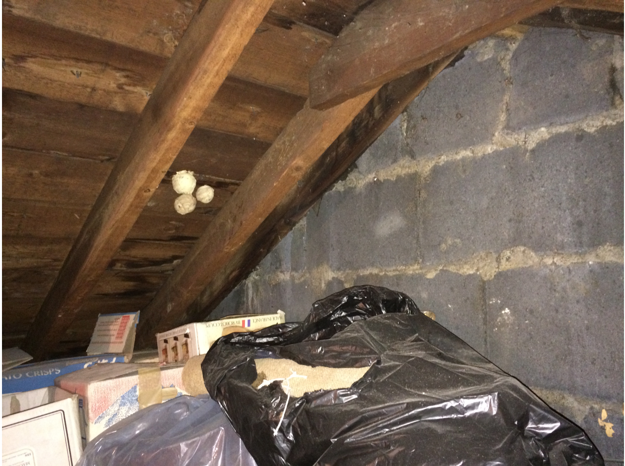
view of rafters at party wall to 21 Keats Grove. Note: party wall rebuilt with concrete blocks confirming repair works have been carried out at roof level in the relatively recent past
