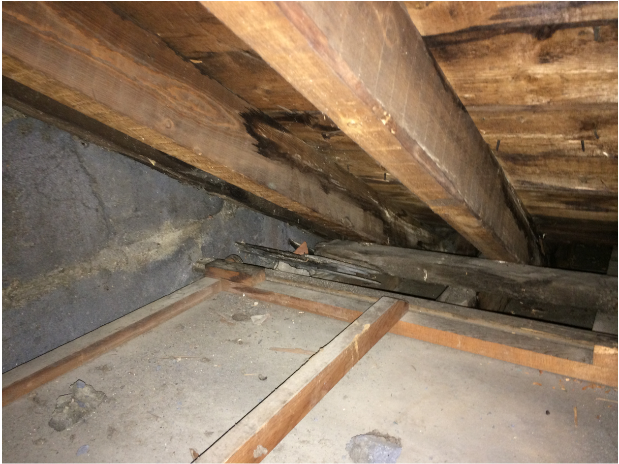
view of rafters at valley gutter showing signs of water staining; note also bandsaw marks on r.h timber.
