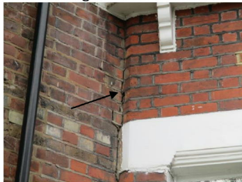
Cracking to front bay
