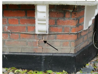
Cracking to front bay
