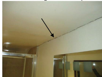
Cracking in flat D bathroom
