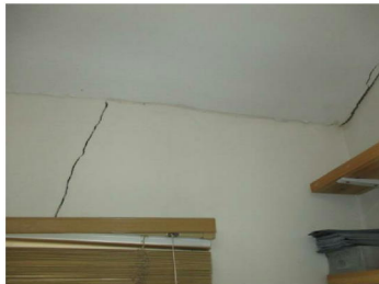
Cracking in flat d above rear window
