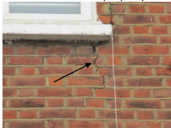
Cracking to front elevation
