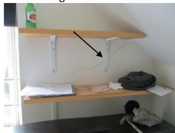
Cracking in flat D front bedroom
