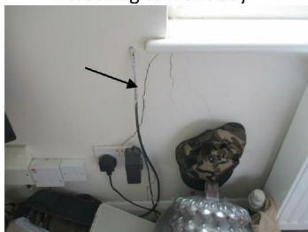
Cracking in flat D front bedroom
