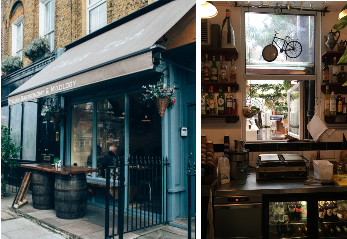
Figure 4 - Existing front access and rear window to be demolished and replaced with a door
