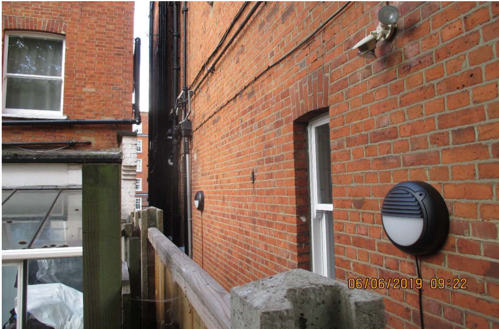
Existing windows in side of adjoining flat alongside four storey building at application site
