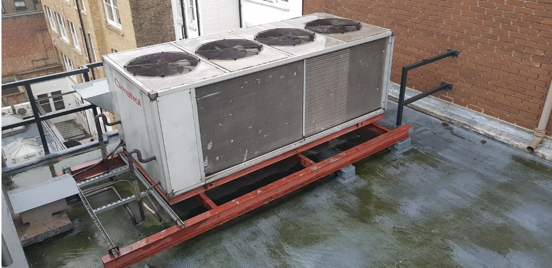
Existing Plant over Fourth Floor Plant Room
