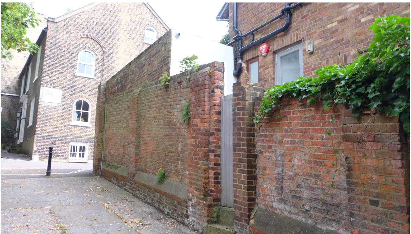
Photo 1 – taken from public footpath running along the north side of the house, looking towards the rear of the existing garage with the boundary wall down the right hand side.
