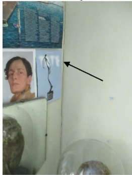
Cracking in 1st floor rear bedroom around rear addition junction
