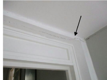
Cracking in kitchen on rear addition junction
