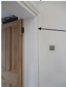
Cracking on 2nd floor landing on rear addition junction
