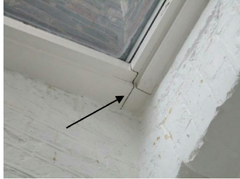
Cracking to glazed roof in kitchen around rear addition junction
