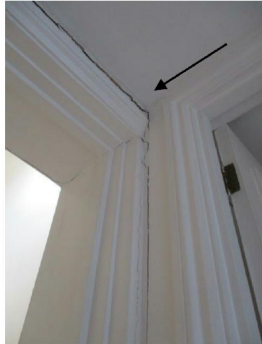
Cracking in 2nd floor rear bedroom on rear addition junction
