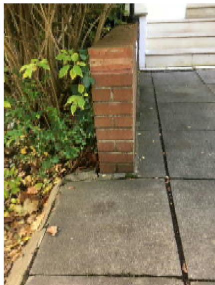
Rotation of dwarf wall at entrance
