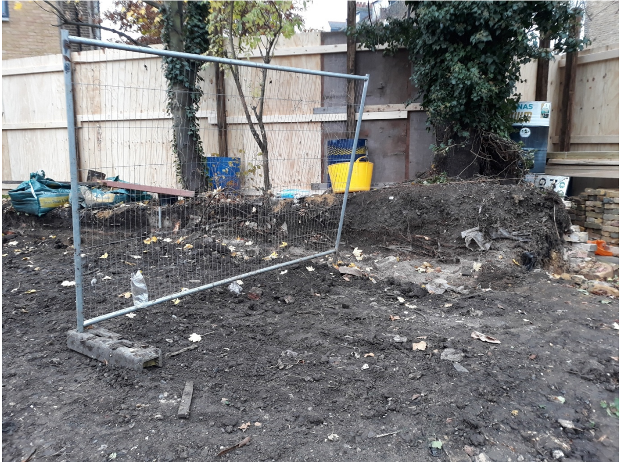
Site Photo 02: A close up of the lime tree root area after removal of existing brick boundary wall.
