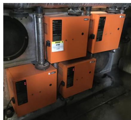
Figure 2 - Existing boilers located in the basement
