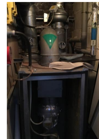
Figure 5 - WC ventilation located in first floor plant room
