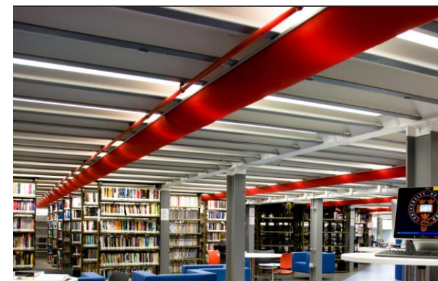
Figure 6 – Ventilation air sock provided within the Bodleian Library
