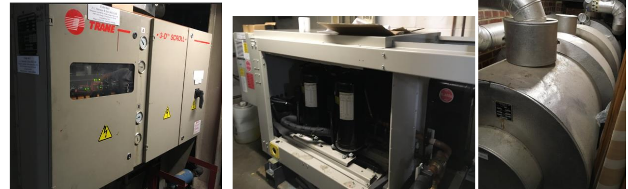
Figure 3 – 2 no. chillers and buffer vessel located in the basement.
