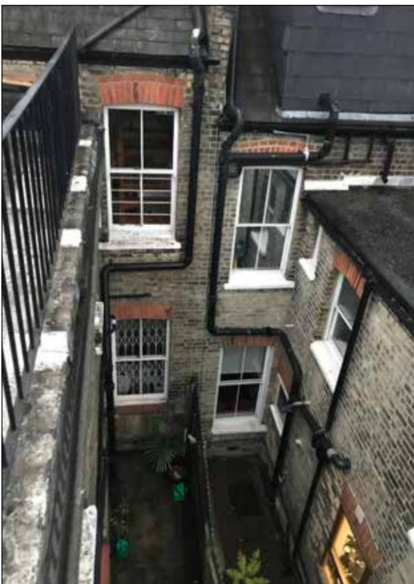
Fig 11. Existing view of side yard from upper floor terrace showing soil pipe serving upper floor - 2019.
