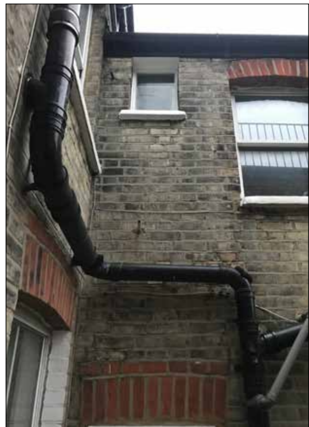
Fig 12. Existing soil pipe from upper floor flat returning over side elevation - 2019.
