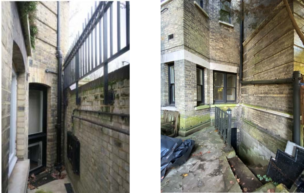
Figure 17 (left) Number 19 shows historic and modern brickwork within the well and traditional brick structural openings.
