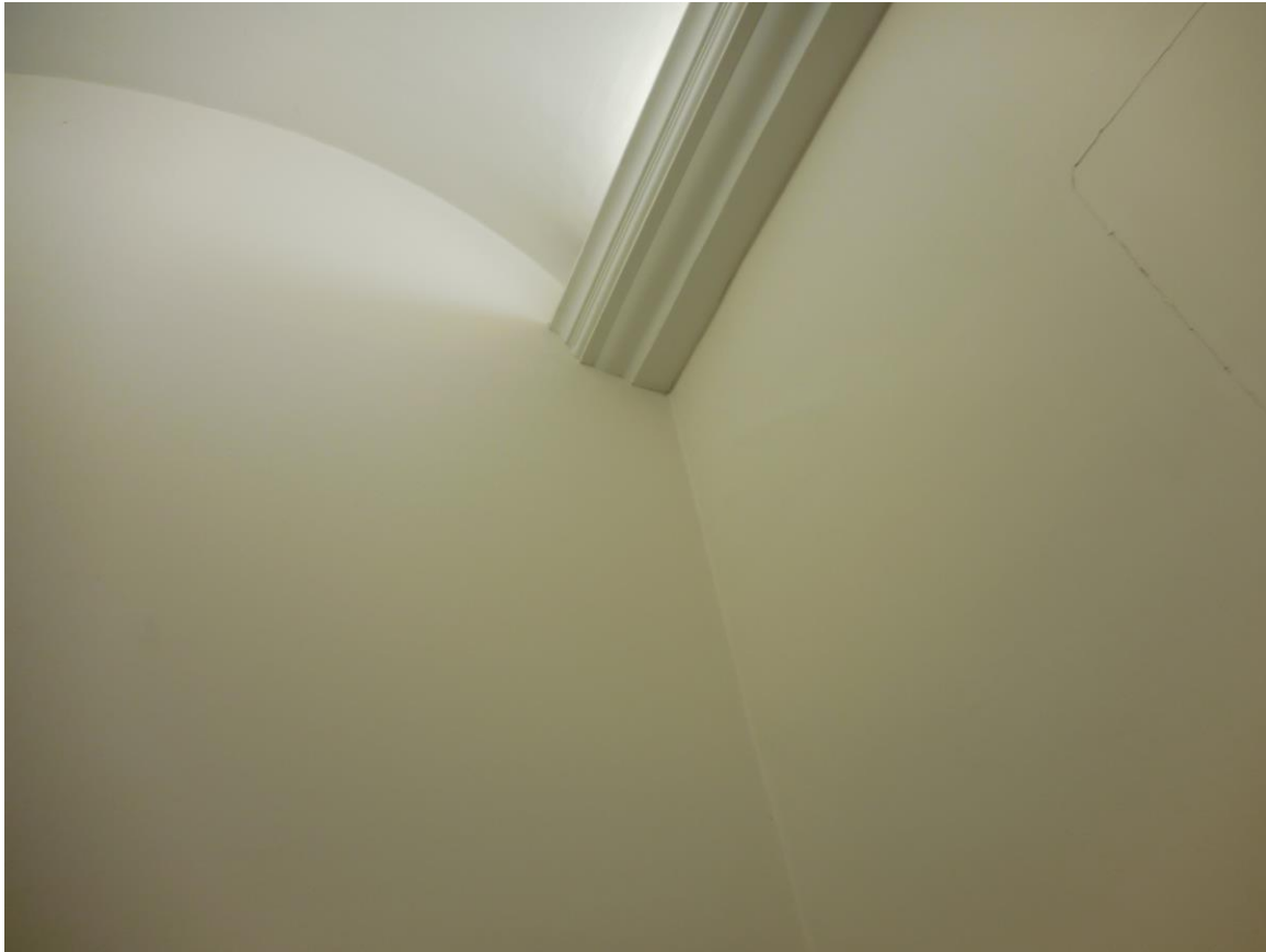
FIG.5 – CRACK LINE IN WALL SHOWING EVIDENCE OF LINE OF ORIGINAL STRUCTURAL OPENING
