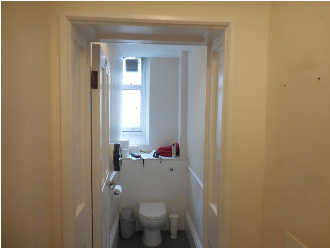
FIG. 1 – DOOR GD-04 TO TOILET. DOOR AND LINING TO BE REMOVED AND INFILLED
