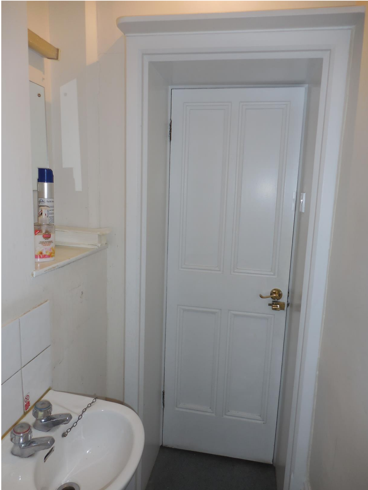
FIG.4 – DOOR DG-03 AND LINING TO BE RETAINED. WASH HAND BASIN TO BE RELOCATED
