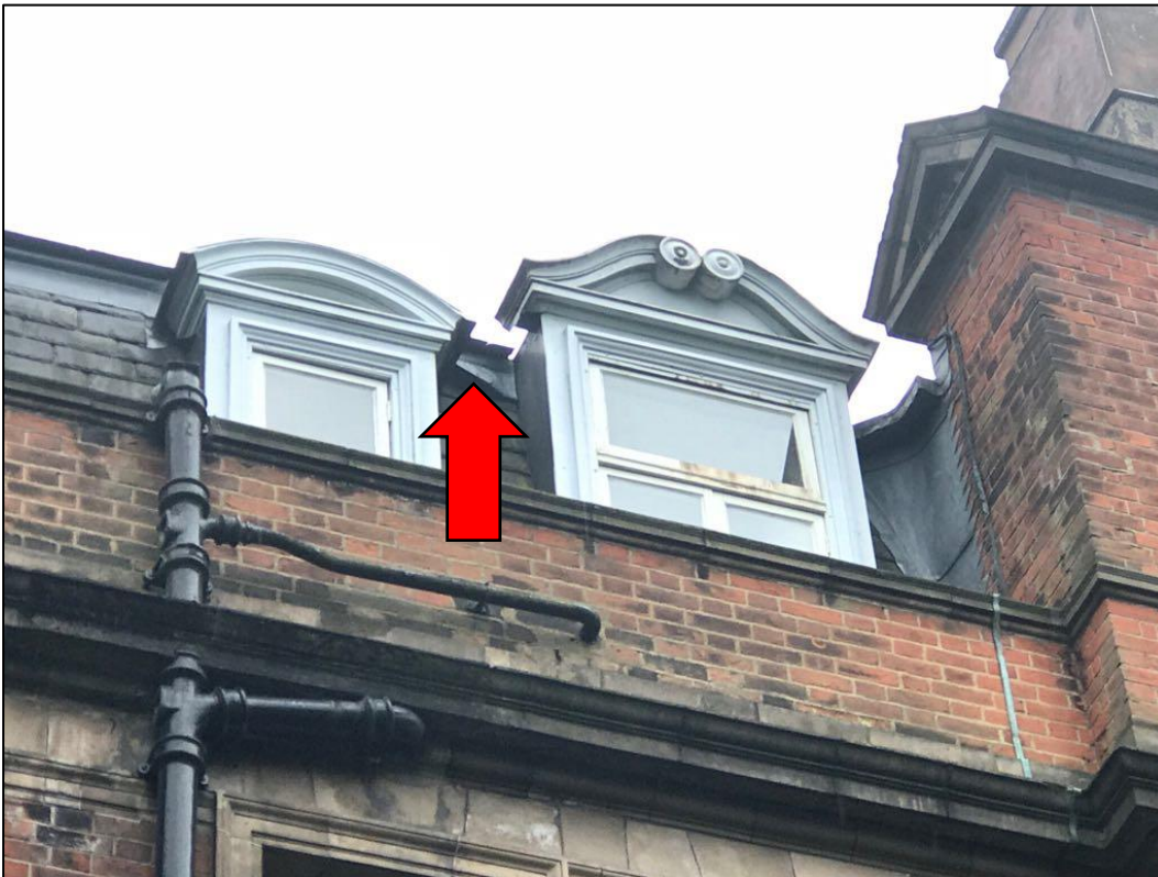
a) B1: Lifted lead flashing next to window
