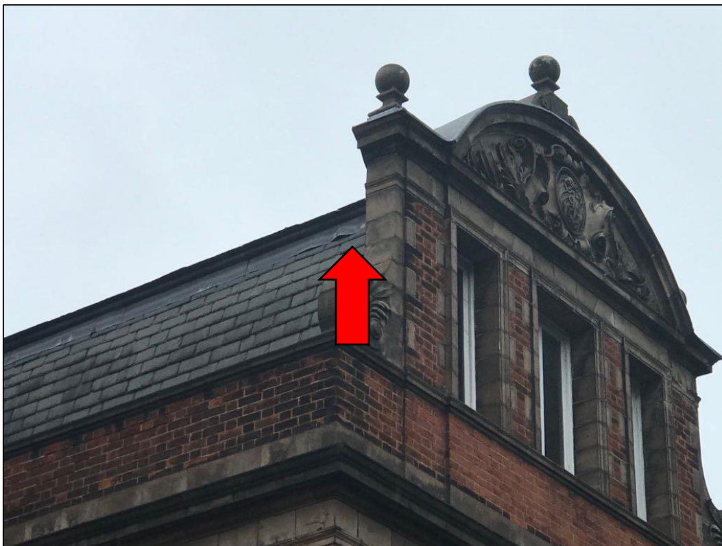
b) B1: Lifted flashing next to ridge
