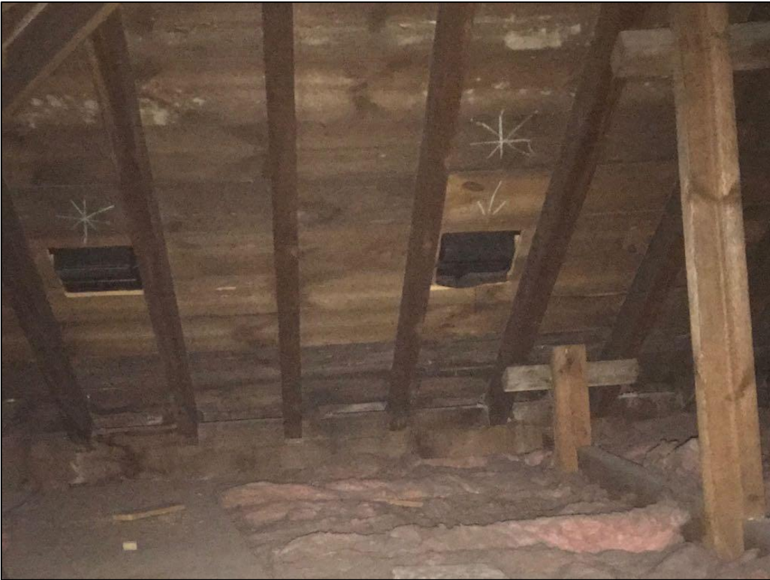
c) Loft vents fitted into loft space in B1
