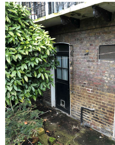
fig 8. Small terrace beneath ground floor balcony is currently unstable
