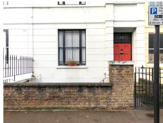
fig 12. Brick wall to street which will be rendered and painted to match the house
