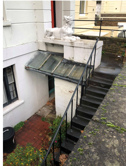
fig 10. Existing unsightly glass roofing with untidy and messy guttering
