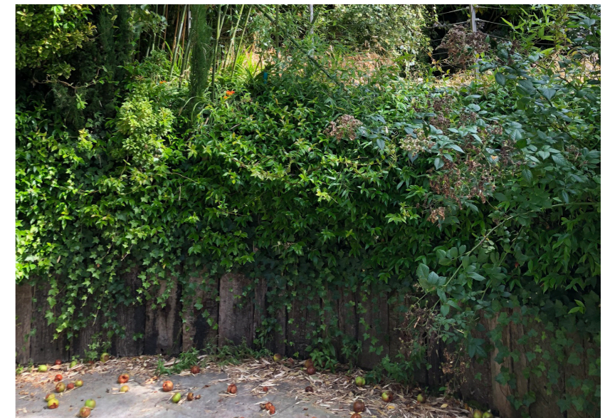
Existing timber retaining wall beneath the apple tree- To be retained within tree root protection area.
