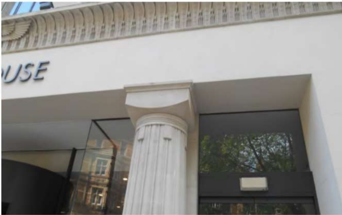
Close up detailing to the front elevation ground floor column and decoration
