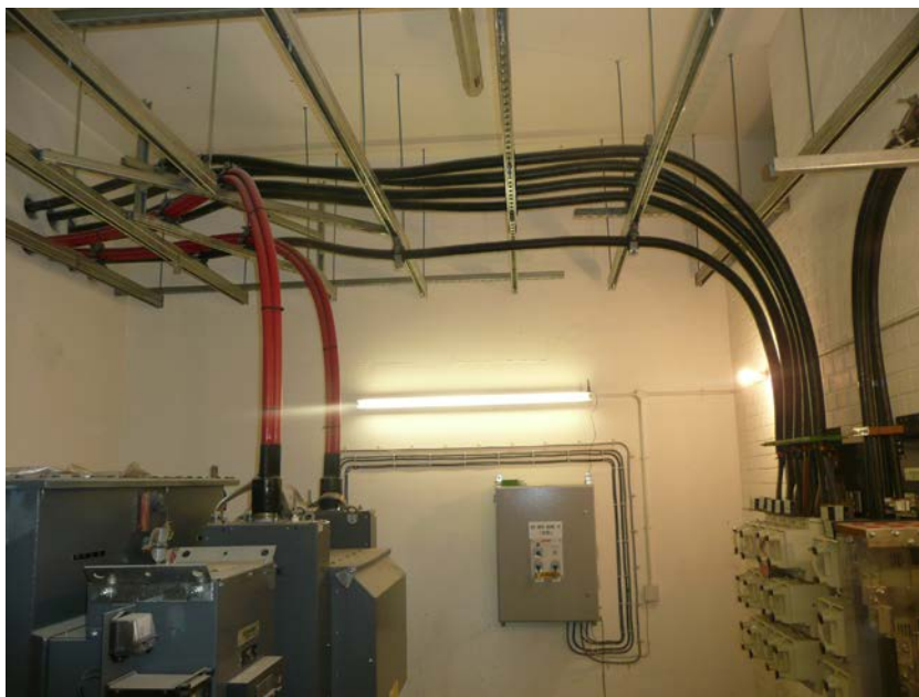
Photo 9: Example of Unistrut 'P1001T' cable supports, allowing cables to be cleared above & below;
