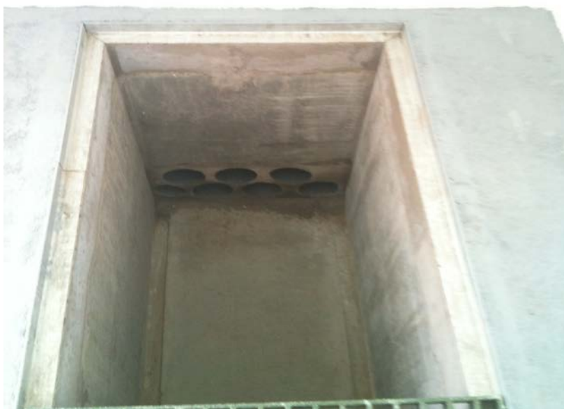
Photo 10: Example of ducts finished flush with the internal face of the substation;
