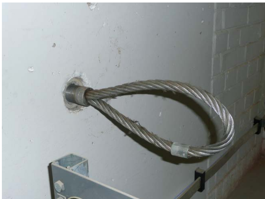
Photo 13: 'Winching eye' for plant installation ~ Example 2;
