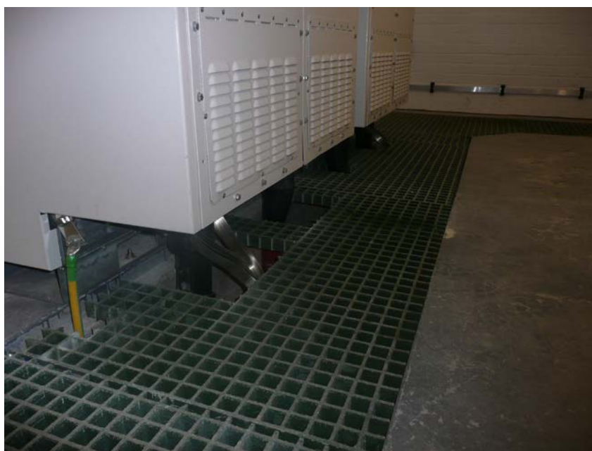
Photo 6: Example of 'cable cut-outs' in GRP grating;
