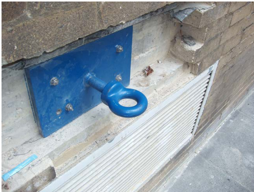
Photo 12: 'Winching eye' for plant installation ~ Example 1;
