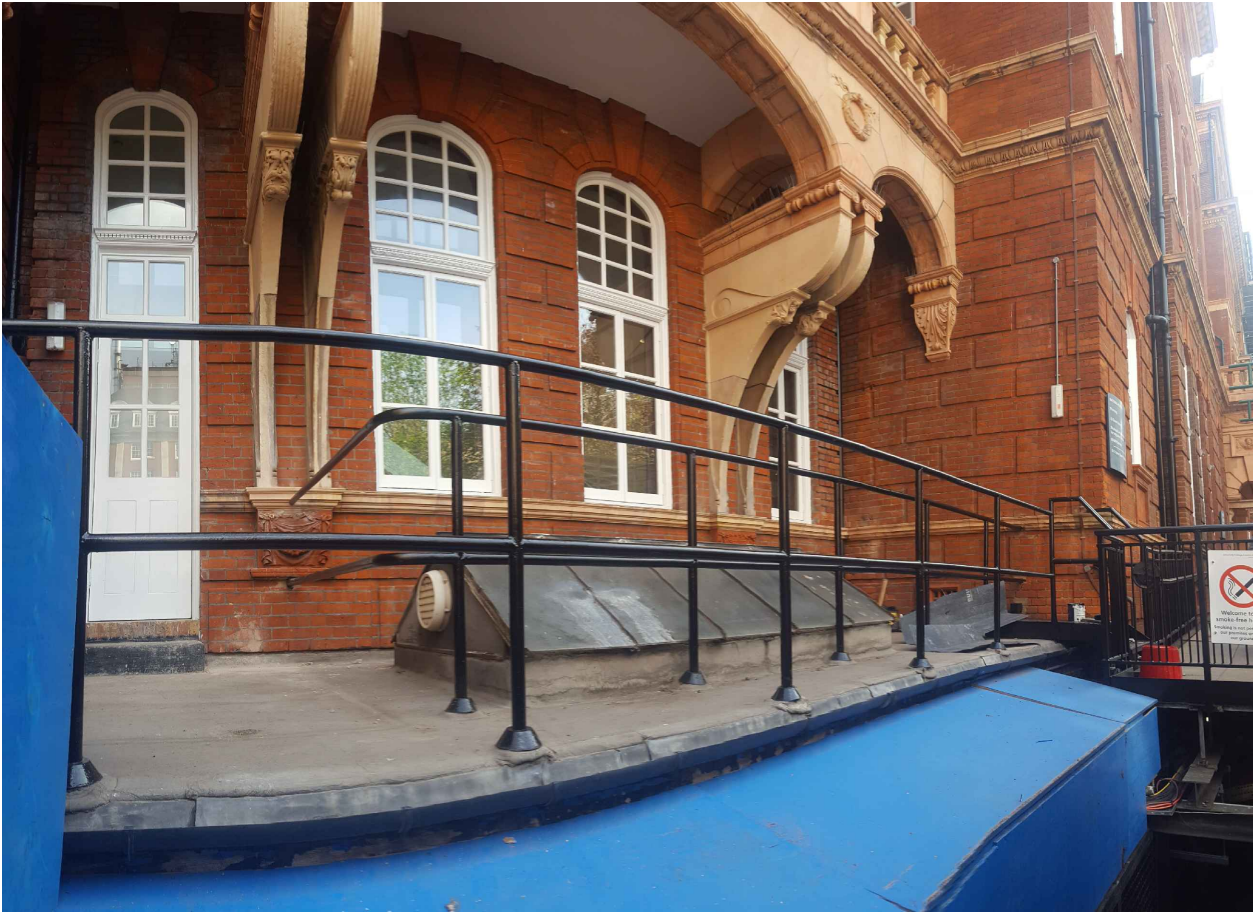
FLAT ROOF BEFORE
