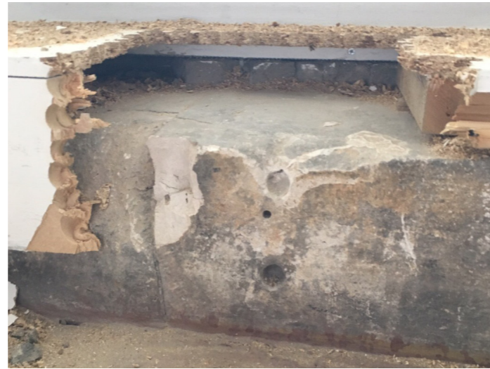
Strip out of boxing at wall where concrete structure projects into room
