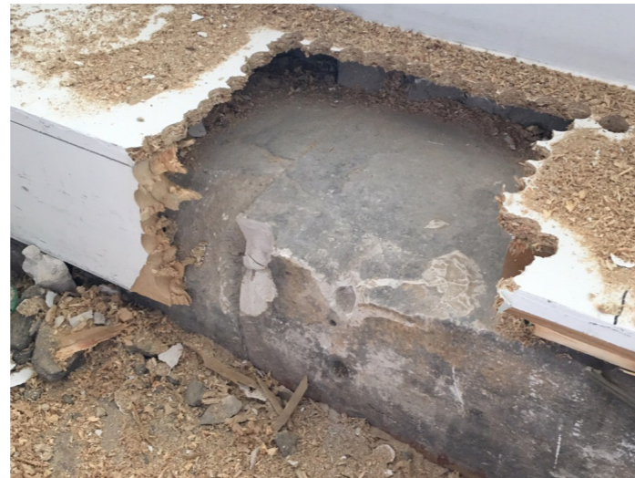
Strip out of boxing at wall where concrete structure projects into room
