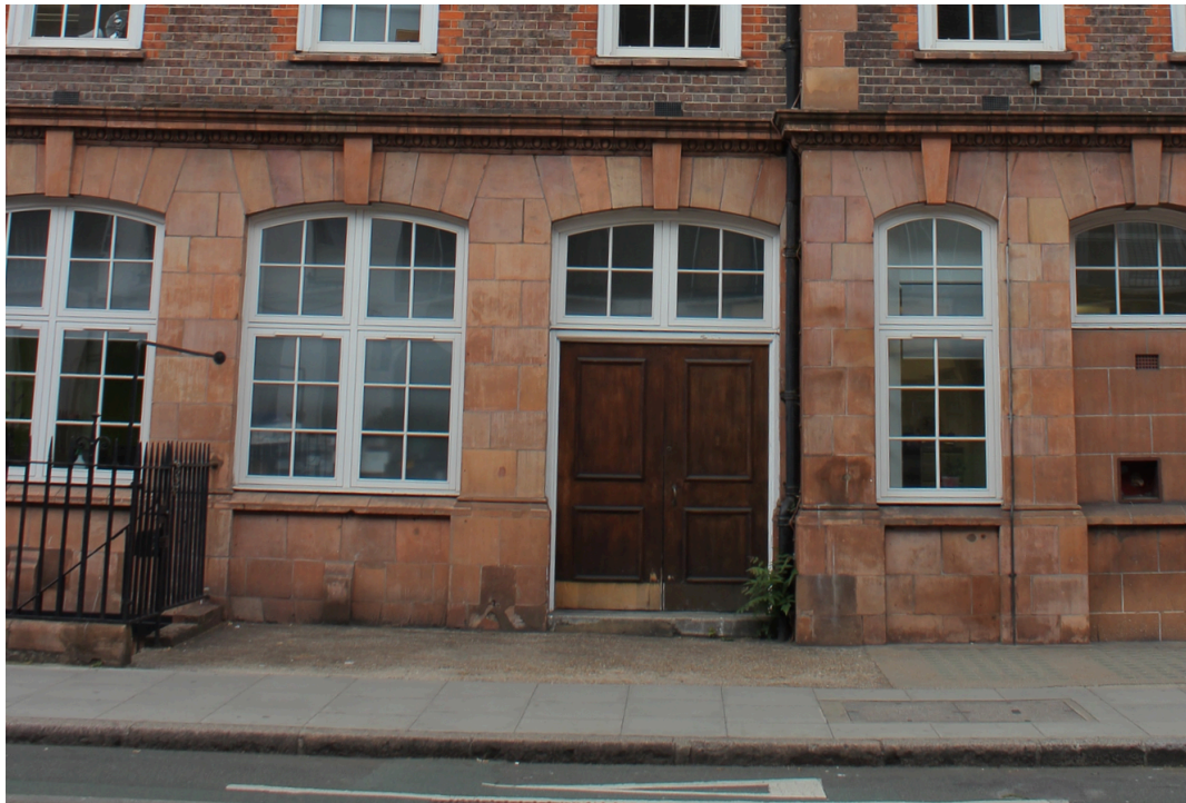
Figure 4: Existing doorway to LSHTM building TP1, to be replaced with new doors.
