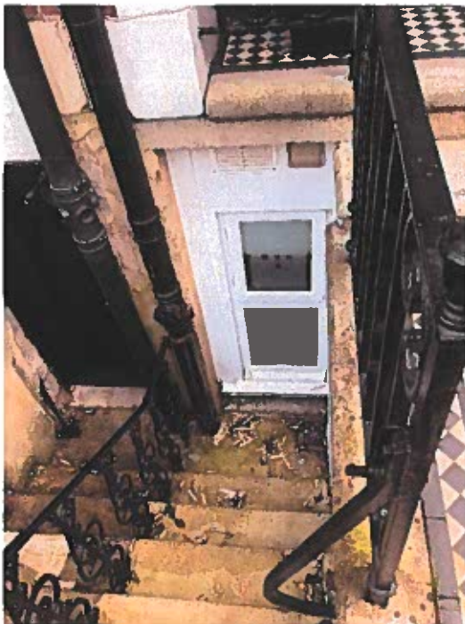
The front basement access stair to be reconfigured and bedroom window cill to be lowered.
