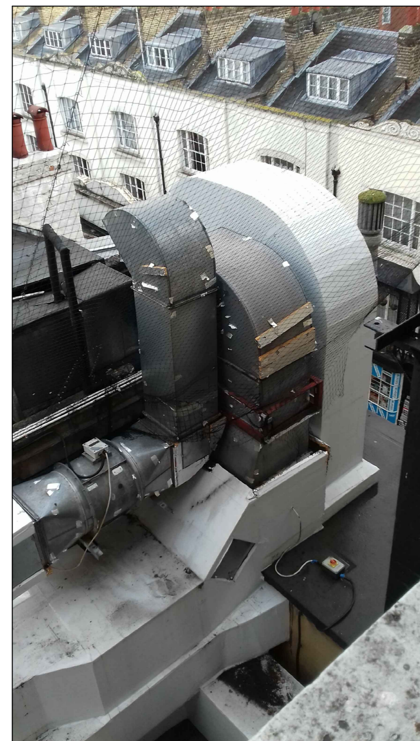
View on existing duct work discharge
